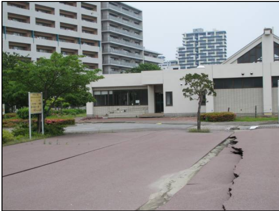
Lateral soil spreading near a community center near Tokyo, Japan, 2011; the pile-supported building survived
