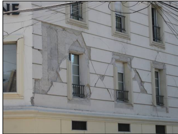
Extensive wall damage in office building in Port-au-Prince, Haiti, 2010, requiring extensive repairs before re-occupancy
