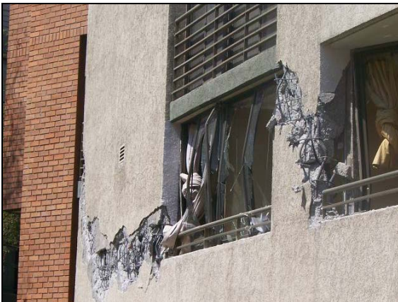
Damaged high-rise residential tower in Santiago, Chile, 2010, requiring substantial structural repairs
