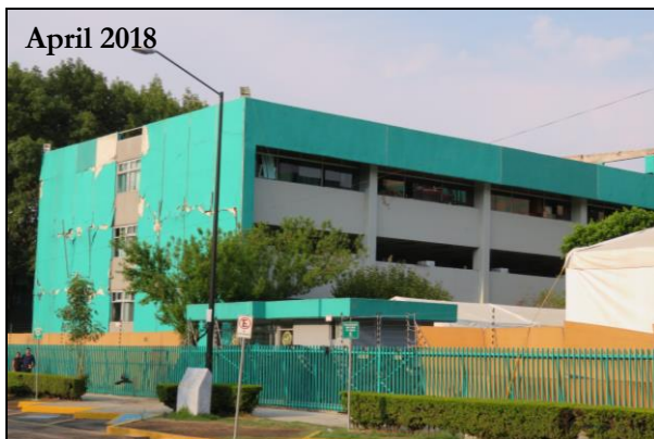
April 2018 Schools: A damaged classroom building still stands vacant at a private college in Coapa.
