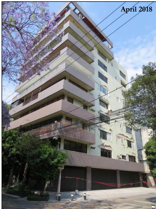
Vacant damaged apartment building in La Condesa. Note concrete frame and brick infill wall construction with extensive ground-level openings.
