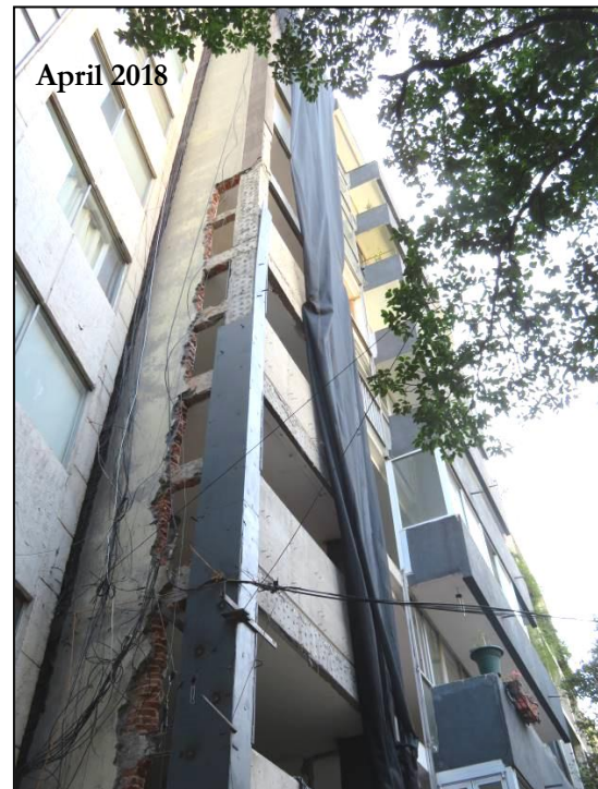
Example reinforced concrete frame apartment building in La Condesa undergoing post-earthquake repairs and retrofit with new steel plates over existing concrete columns.
