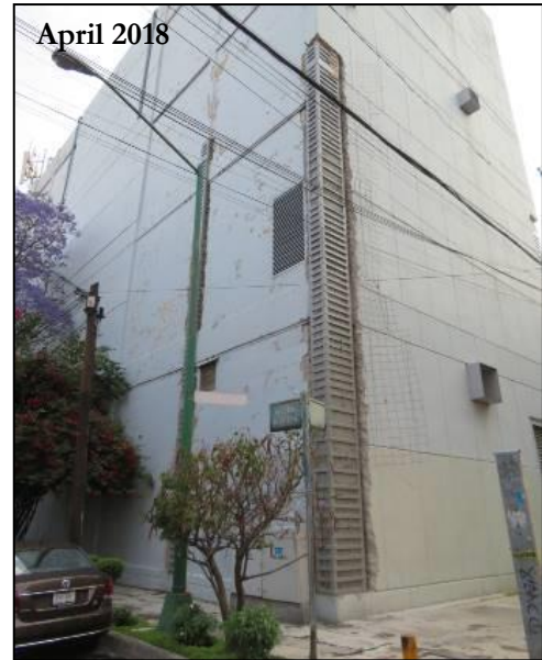
April 2018 Critical facilities: Earthquake repairs and upgrades (column strengthening) continue at a telecom central office in Coapa.
