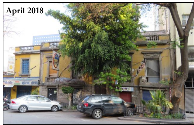
April 2018 Vulnerable structures: A damaged unreinforced masonry (URM) building (adjacent to a high-rise apartment building) remains unattended.
