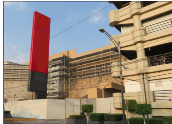
Earthquake damage repairs still in progress at the Coapa regional shopping mall.
