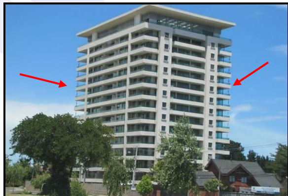
Damaged condominium tower in San Pedro still stands vacant. Corner balconies remain shored up.
