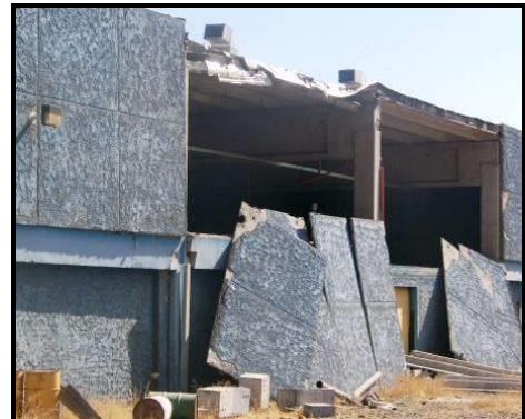
Precast reinforced concrete construction at Ciudad Empresarial. Inadequate wall panel connections resulted in building damage.
