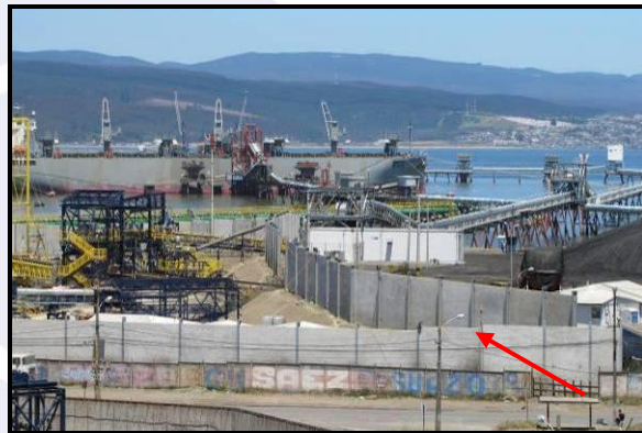
Low-lying areas of Port of Coronel (south of Concepción) are surrounded by newly constructed flood walls.
