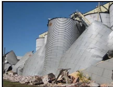
Collapsed thin-walled steel grain tanks.
