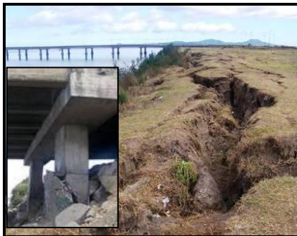
Juan Pablo II (Concepción) bridge damage and riverbank lateral spreading.
