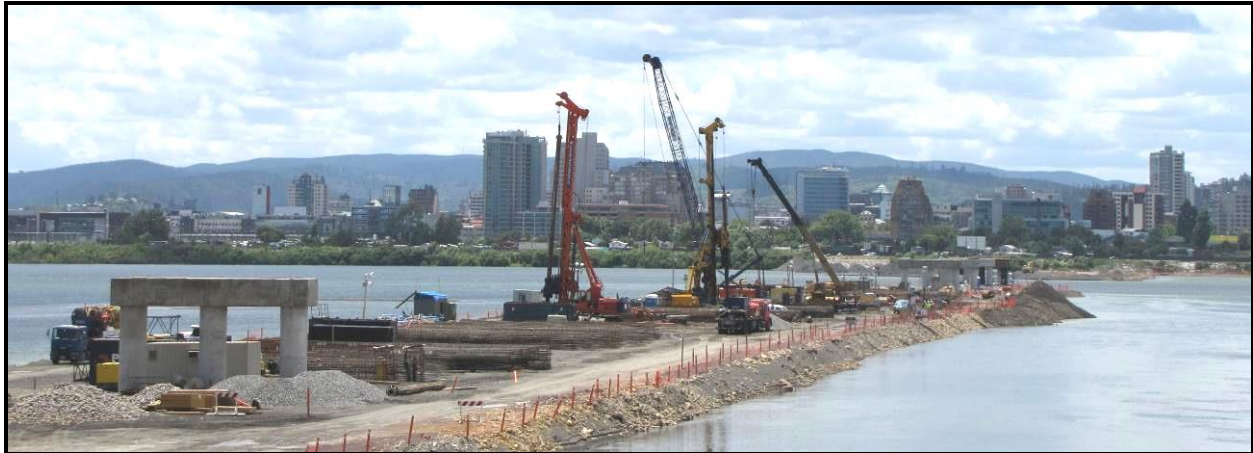
December 2010: Construction is in progress on a new highway bridge over the Bío Bío River in Concepción. This crossing will replace a bridge damaged by the earthquake. The city skyline (background) includes a number of vacant residential towers.
