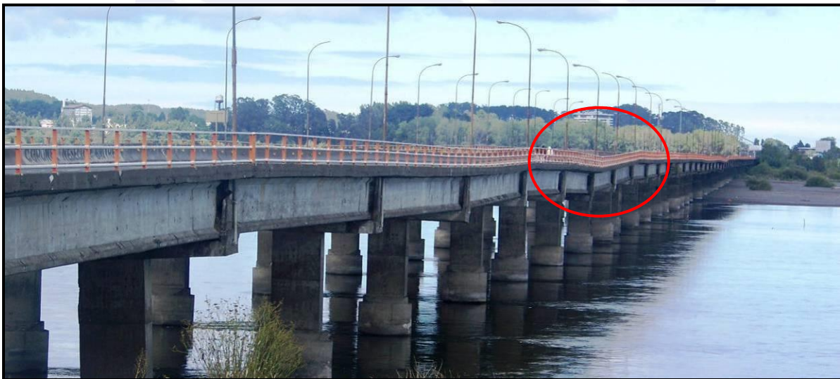
Juan Pablo II Bridge damaged in the February earthquake was restored to service in October 2010. This photo from March 2010 illustrates some of the bridge foundation damage as evidenced by the sagging roadway.
