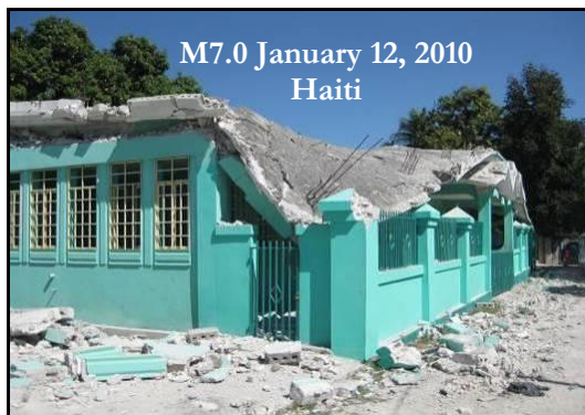
Second-story collapse in a newly constructed hospital in Santo, Haiti
