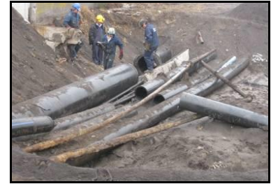
Soil impacts: repairs of piping damaged by soil liquefaction
