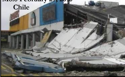
Collapsed concrete tilt-up wall panels due to weak wall-to-roof connections
