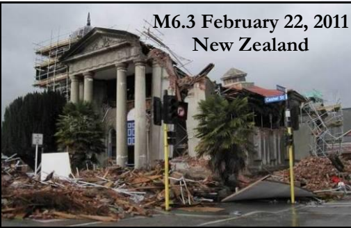
Collapsed unreinforced masonry structure in Christchurch
